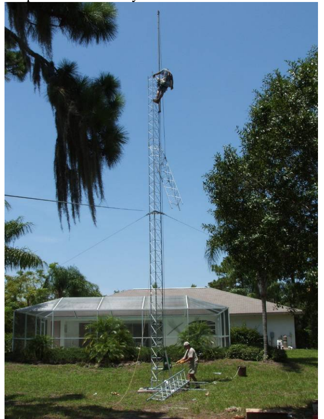
The morning of 04 August, Ron's at the 40 ft. level as Julio hoists up the next section. The first set of 1/4" EHS guy wires are attached 21 ft. above ground.
