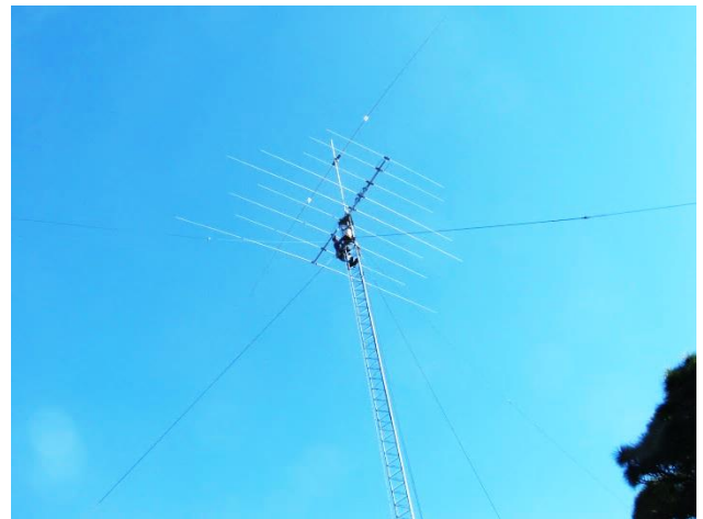
Ron LeBrun-KB4RON replacing the rotator on the 80' Rohn 45 tower at the Radio Cottage of Al Culbert-K0AL.
