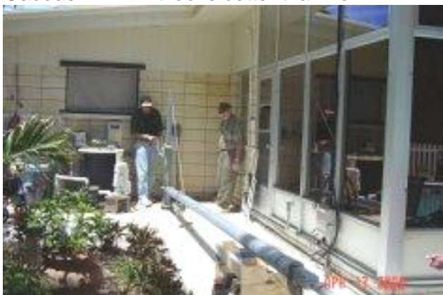
The telescoping, two-section tubular tower is attached and just starting to rise up from its supporting cradle. Note Bob-N1RA providing moral support. When completed, Jack will have a two-element home-brew cubical quad at the top of this tower.
