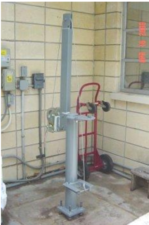
Here's a shot of the completely refurbished base and raising fixture for the US Towers MA40 tubular tower being installed at the QTH of Jack Gaddas-KY1Z. It looks better than new!!
