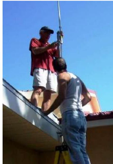
Andy Durette-KB1HIP is shown installing the new antenna at the Sarasota DARN station this past May.
