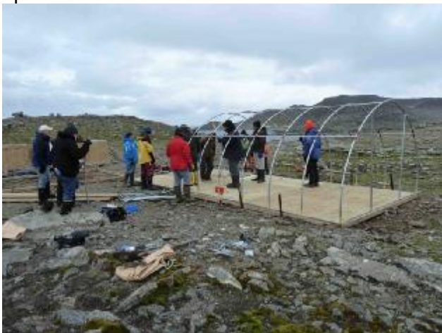
Erection of one hut begins. The team had practiced assembling these arctic weather-
